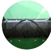
Ripped belt for feeder or fine fraction
